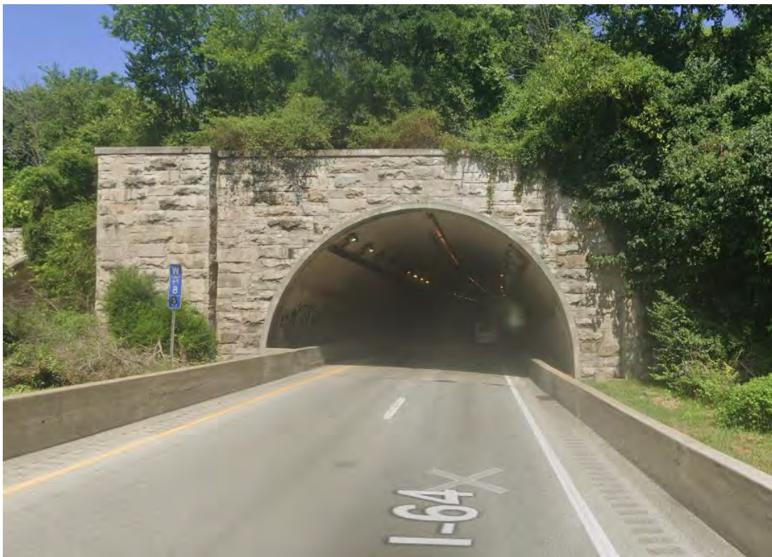
Photo No. 8 – View of east portal for WB lanes at Cochran Hill Tunnel
