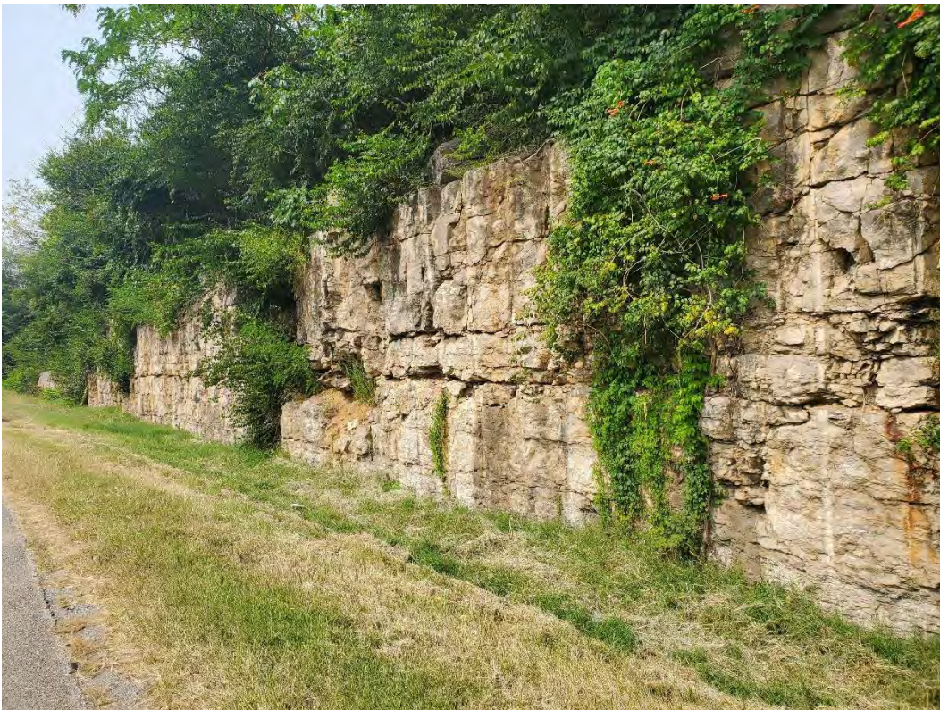
Photo No. 4 – View of rock cut along WB lanes near Breckenridge Lane overpass
