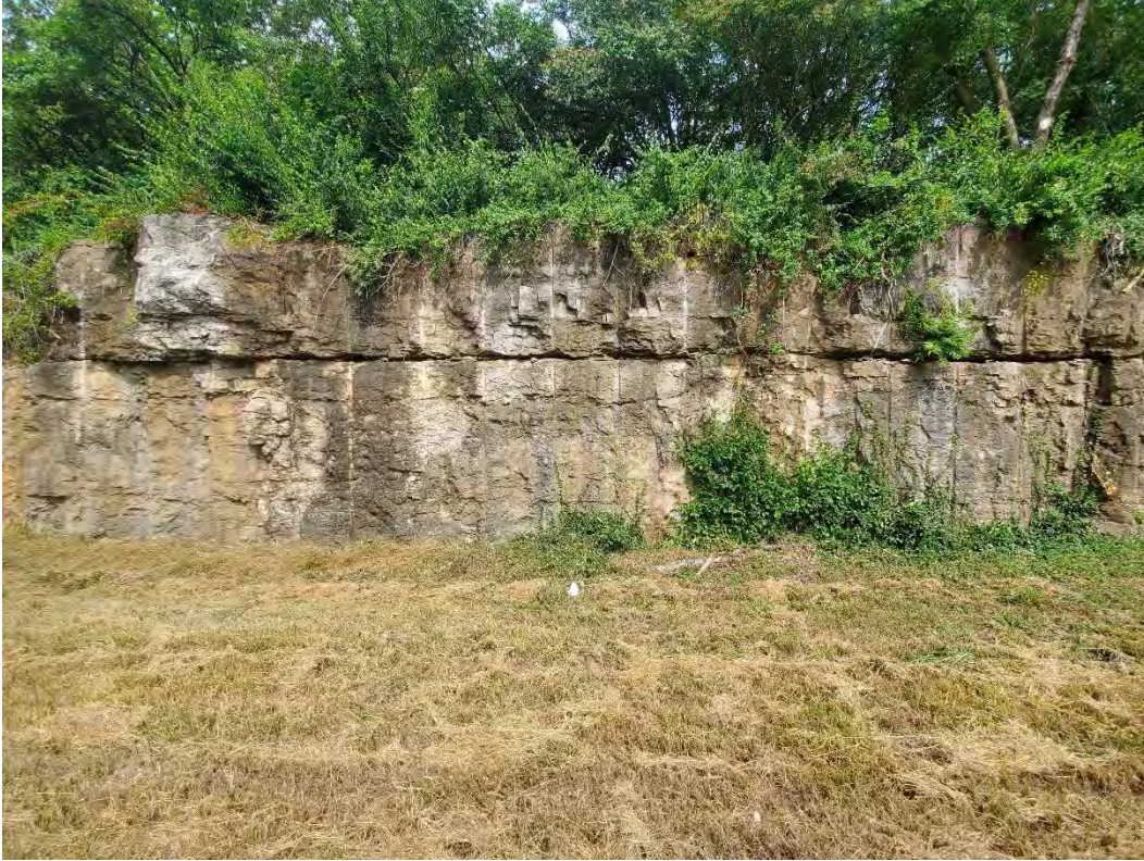
Photo No. 5 – View of rock cut along WB lanes near Pee Wee Reese Road
