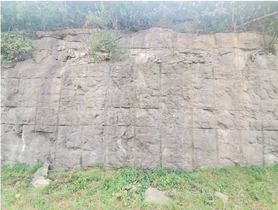
Photo No. 6 – View of rock cut along EB lanes near Beals Branch Road
